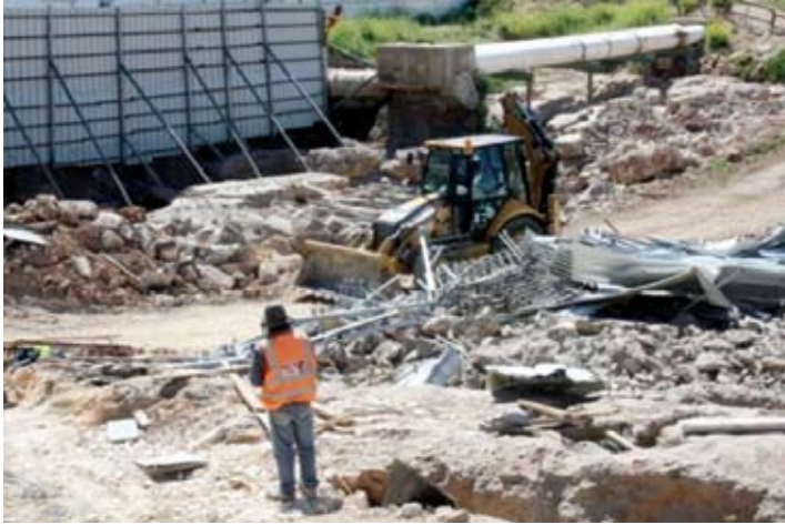
Photograph 5: Heavy earth moving equipment is being used on the site, despite the continued presence of archaeological and human remains throughout the site.
